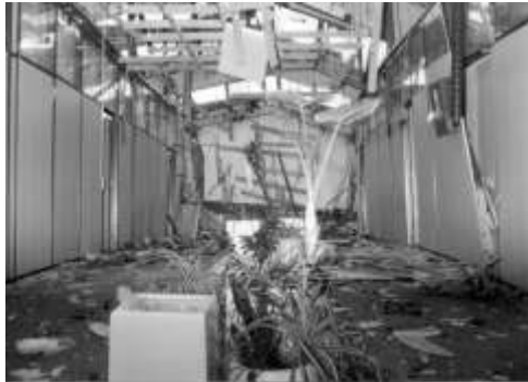
IT building after ATO attack
